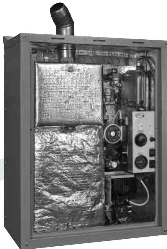
Figure 1-2: Boiler front panel removed
