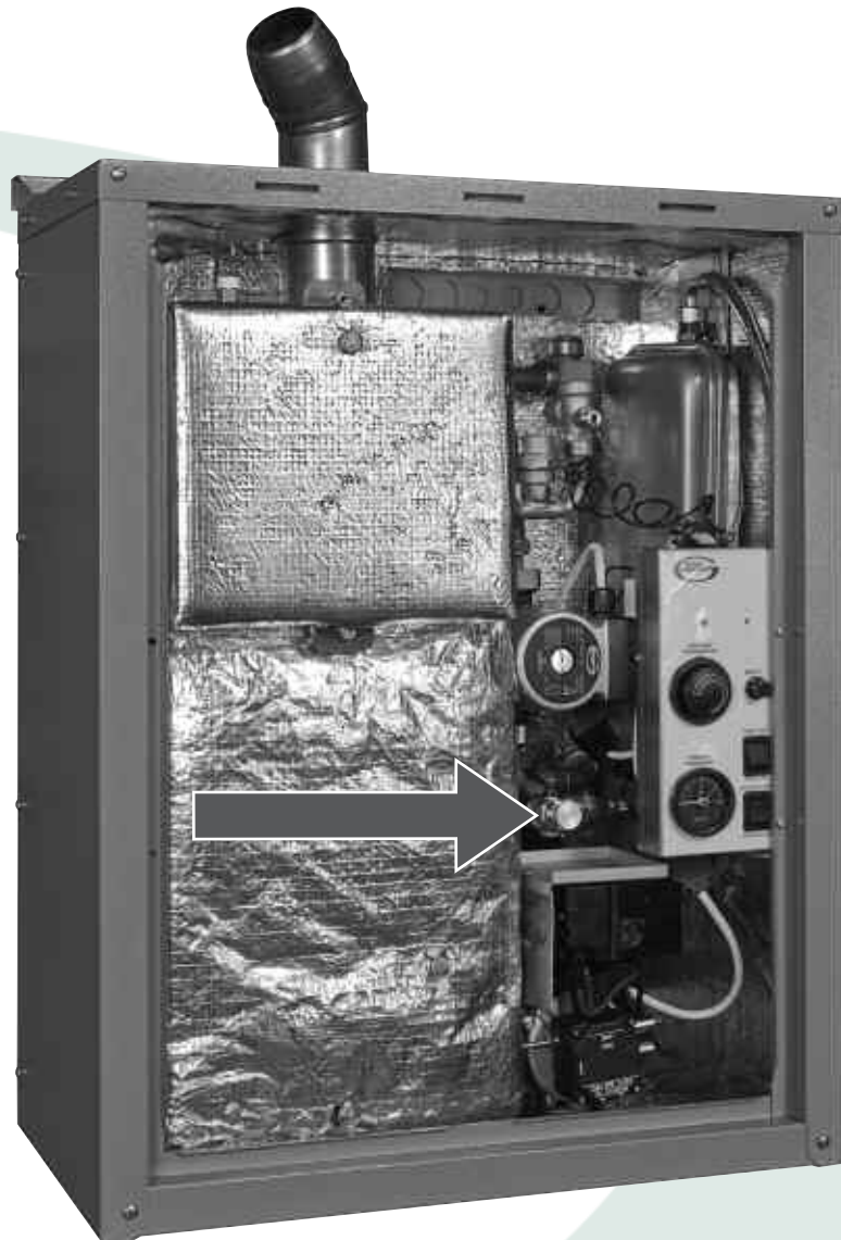
Figure 7-4: Position of water supply valve
