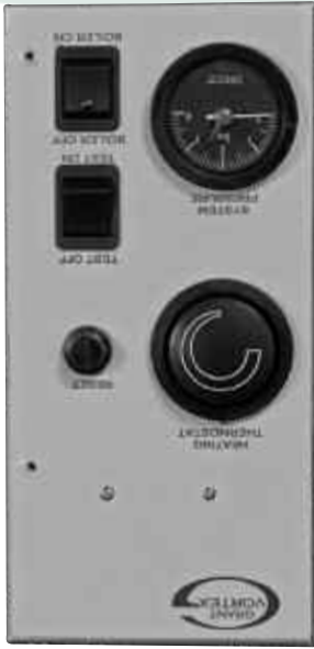
Figure 3: Boiler control panel
